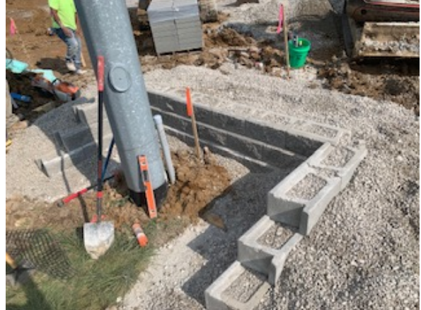
Protecting the Mass Notification Tower
