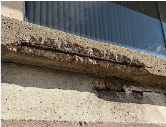
Spalled concrete slab edge/exposed rebar
