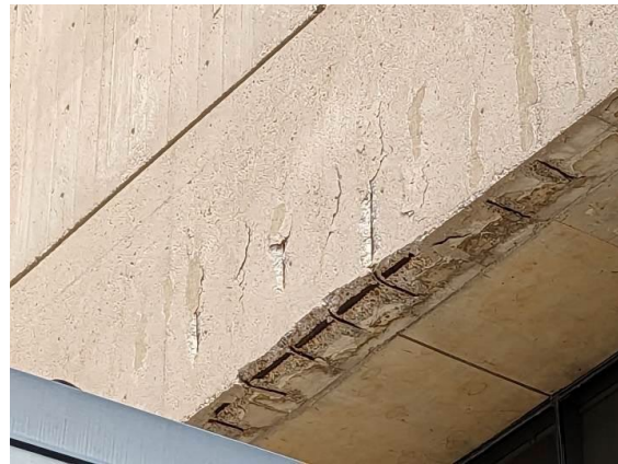
Concrete vertical surface spalling
