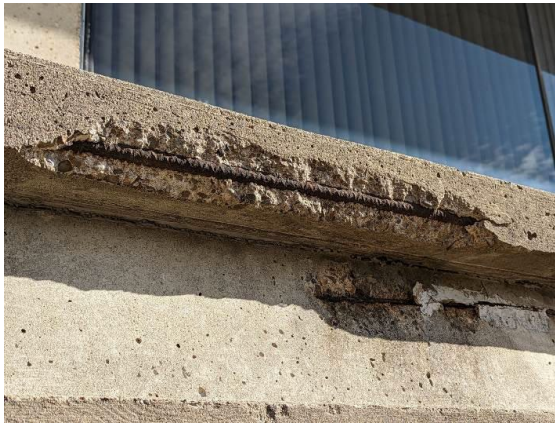
Spalled concrete slab edge/exposed rebar
