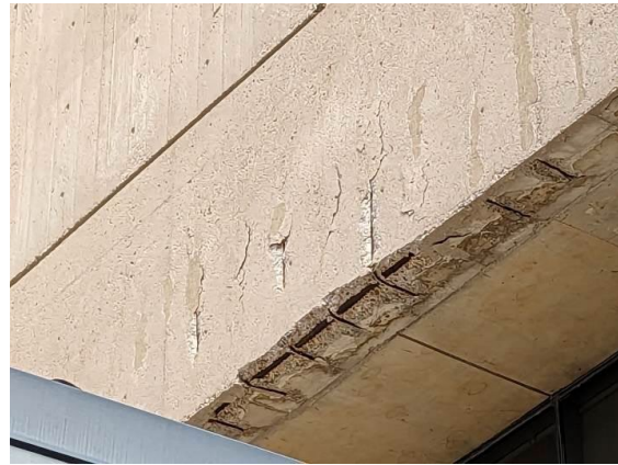
Concrete vertical surface spalling
