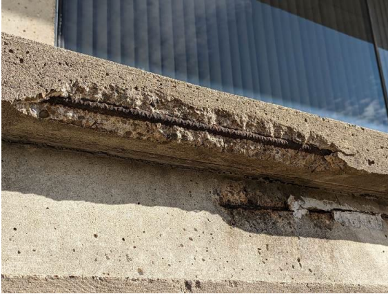
Spalled concrete slab edge/exposed rebar
