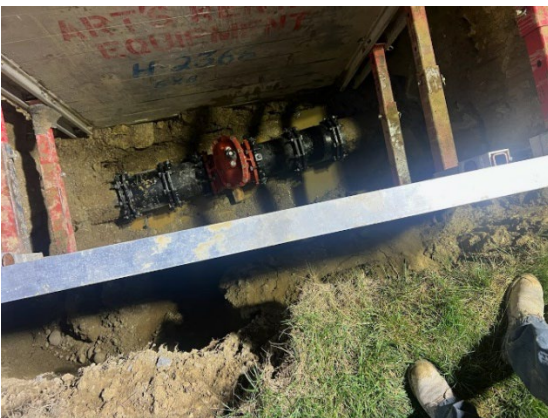
Replacement Water Valve
