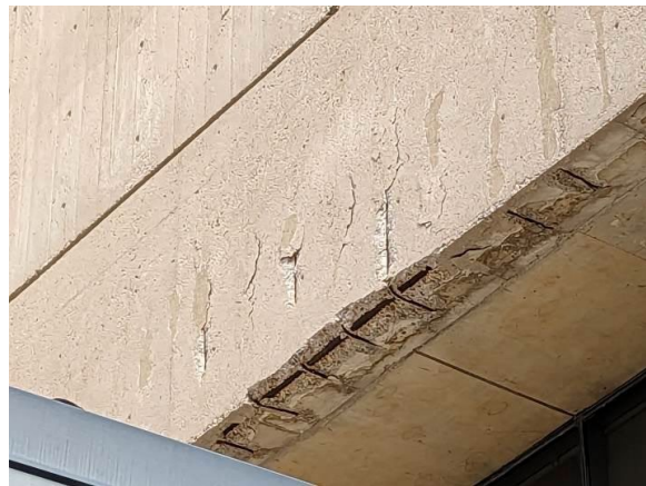
Concrete vertical surface spalling
