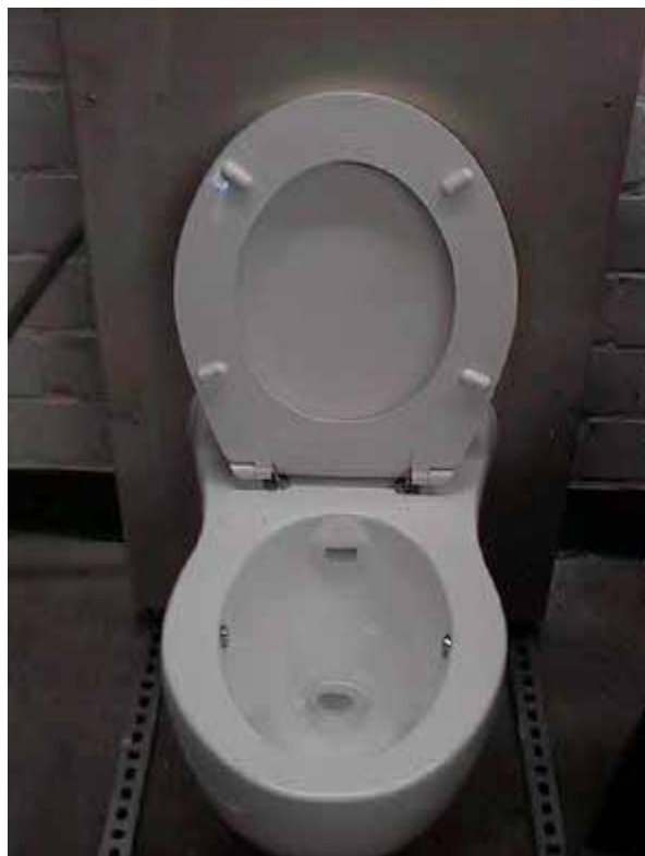
Fig. 3: Vacuum-toilet flushing with approx. 1 l per flush
