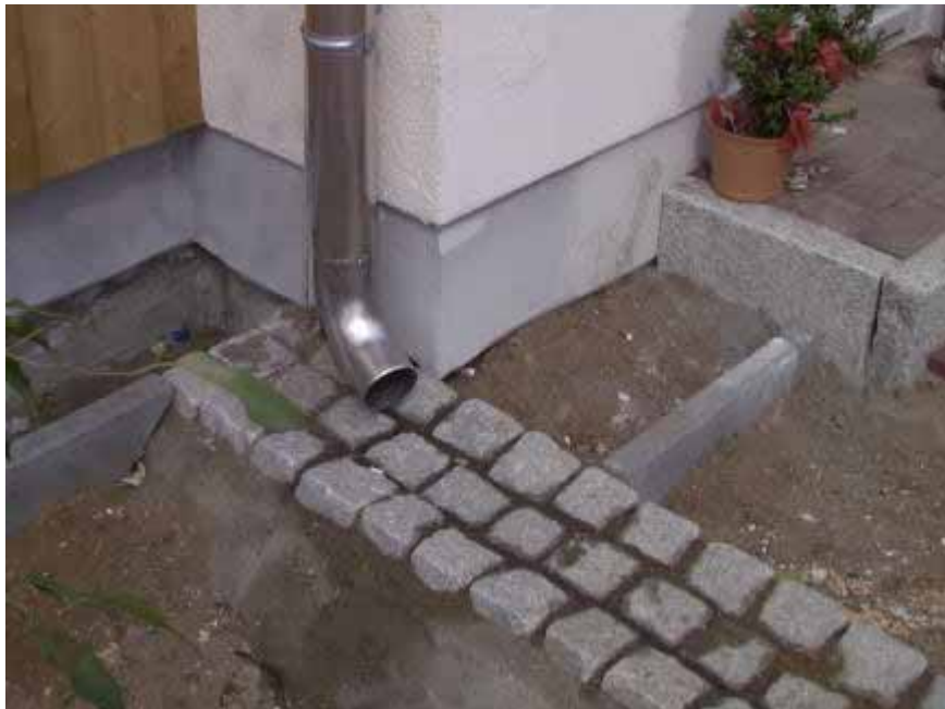
Fig. 5: Gutter for the transportation of stormwater
